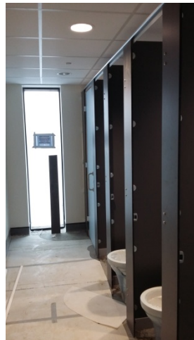
Work ongoing to install the IPS and WC's in the pupil toilets
