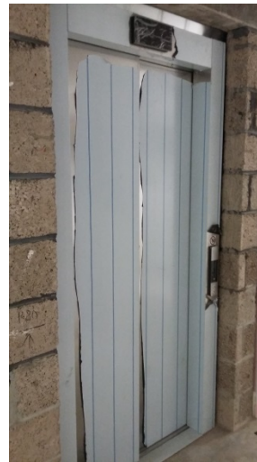
Lift installation awaiting commissioning
